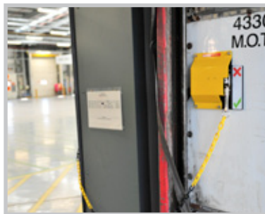
5. Trailer brakes are now applied & the driver cannot move the vehicle. Loading can commence.
